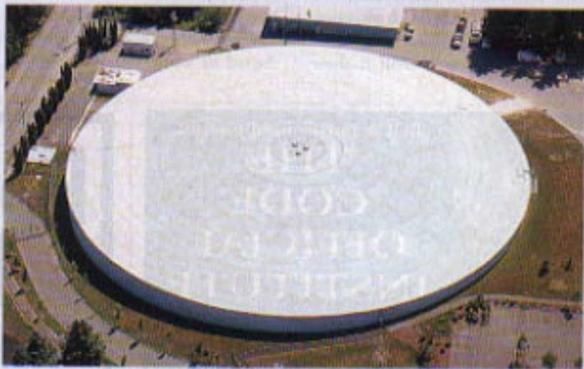
During the cover's construction, the roof frame rested on a 218-foot tower while workers installed stainless steel support columns underneath it.
